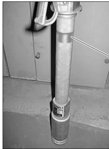
Indication for a Blown Fuse
