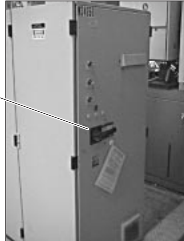
Main Laser Disconnect
