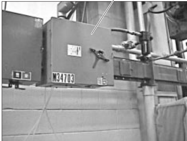
Chiller Buss Plug
