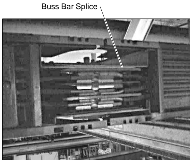
"Breaking" the Buss Bar Splice
