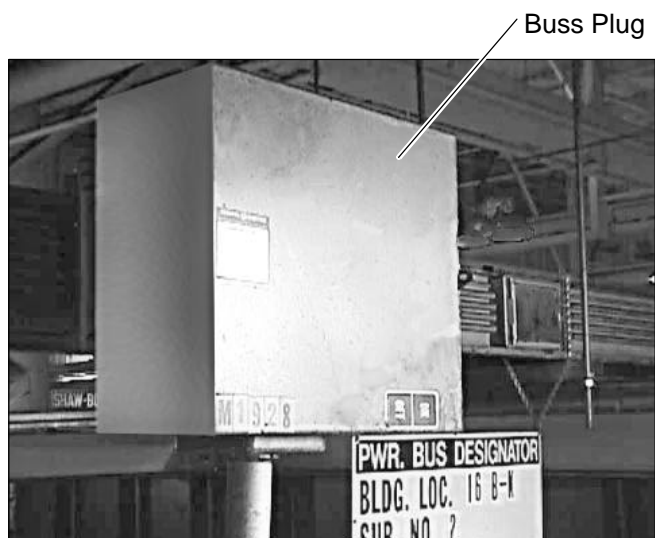
Disconnect and Support Buss Plugs and Conduit
