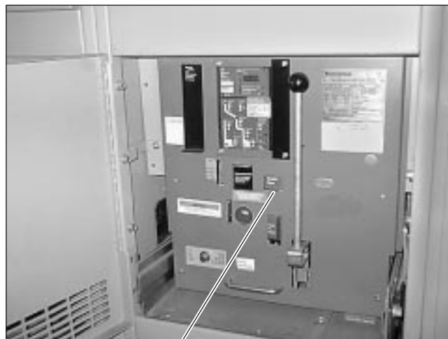
Breaker Status Indicator
