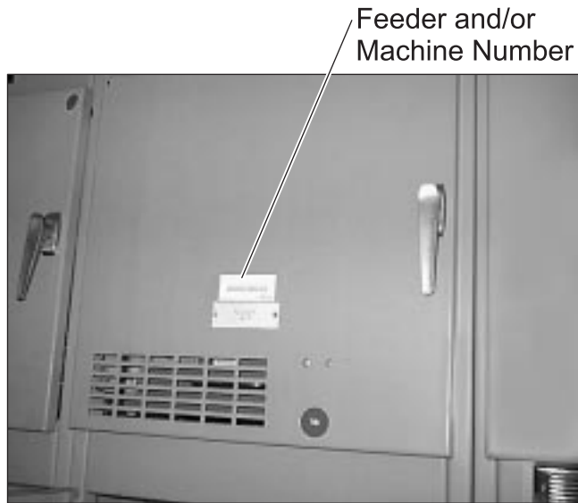
Substation Breaker Identification
