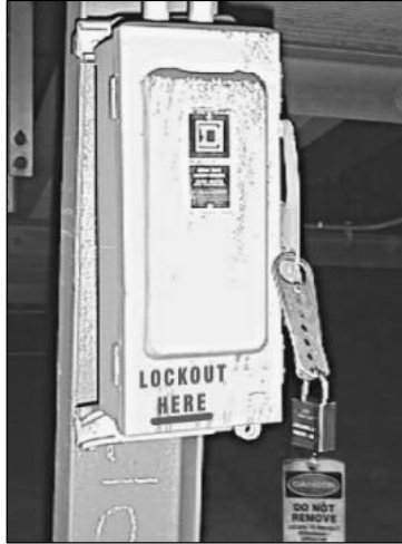
Crane Power Supply Locked Out and Tagged
