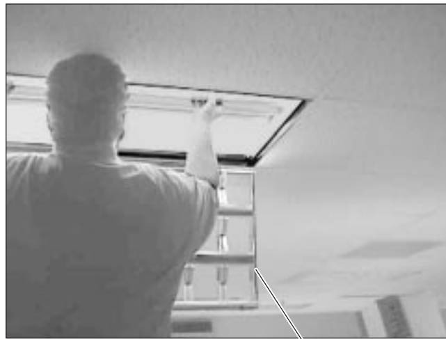
Lowered Light Fixture
