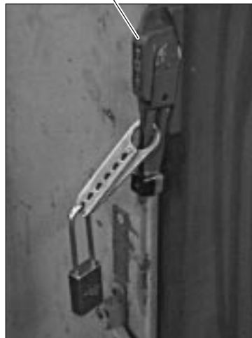
Main Power Disconnect
