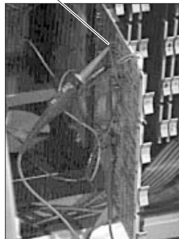
Measuring Voltage on Back of Board
