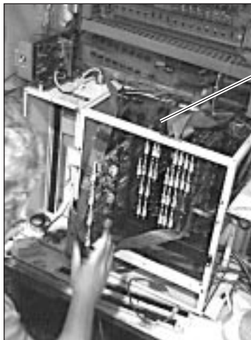
Board Installed with Extension Cards
