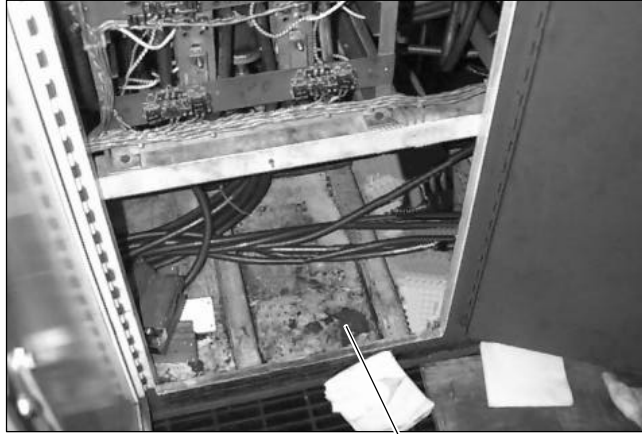
Check for Water Leakage
