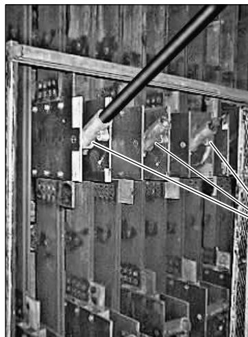
Knife Switches in the Open Position
