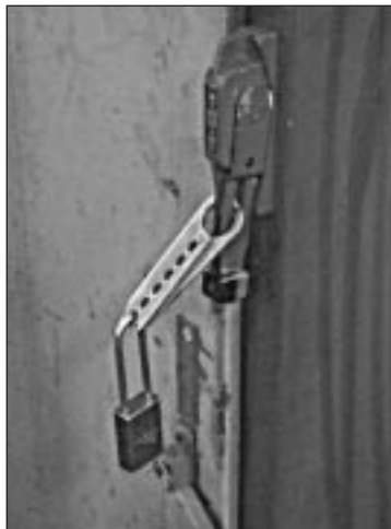
Locked Out Power
