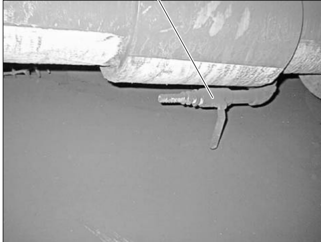
Drain and Vent Valve
