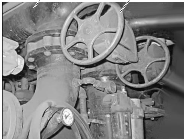
Furnace Water Valves
