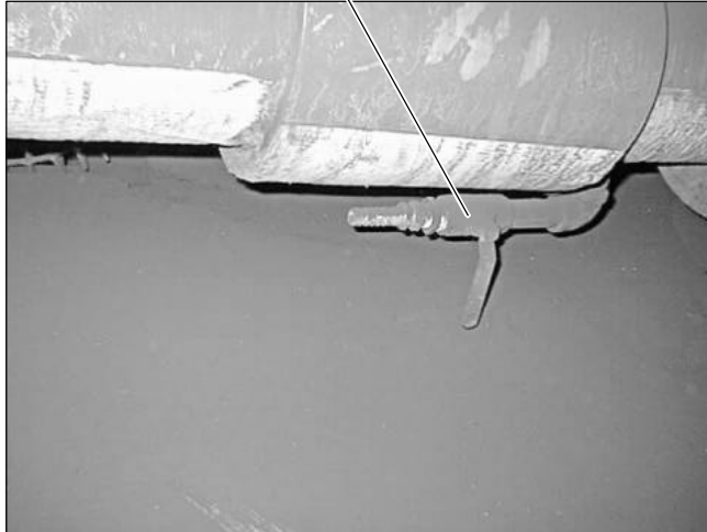
Closed Drain Valve
