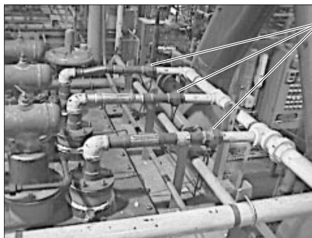
Gas Pipe Unions
