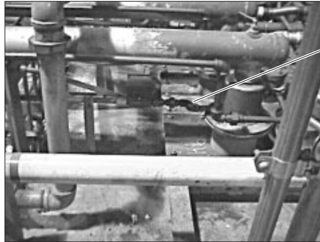
Water Supply Pipe Union
